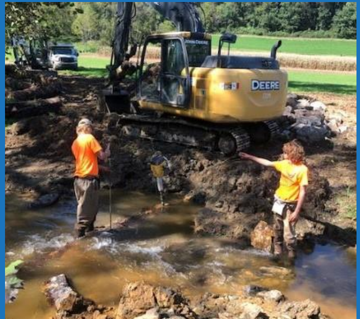
USFWS builds a mudsill to stop severe erosion, reduce pollution, and improve aquatic habitat on Climbers Run.
